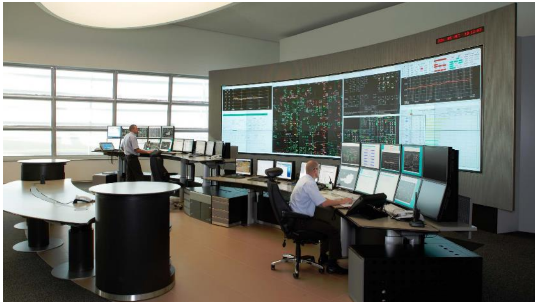
Picture: Lukas Dostal / Austrian Power Grid AG (APG Control Centre)
